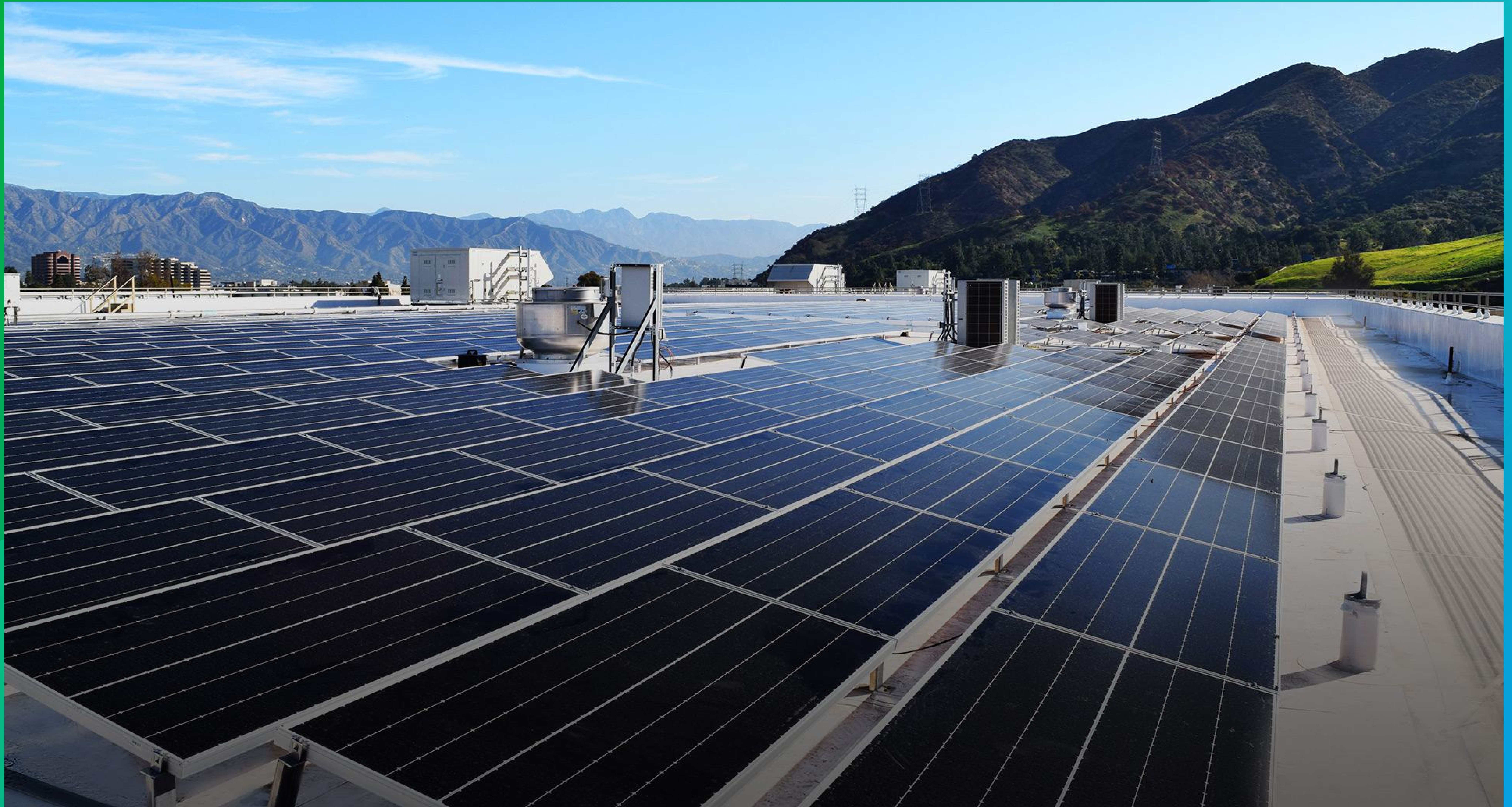
On-site solar at the Universal Studios Lot in Los Angeles
